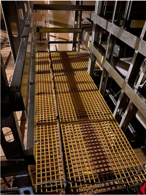
Expanded catwalks in the mezzanine
