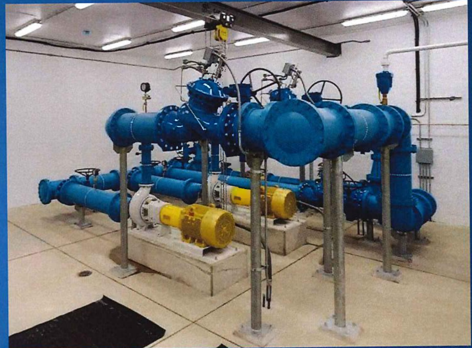
Picture: Manchester Road Booster Pump Station
