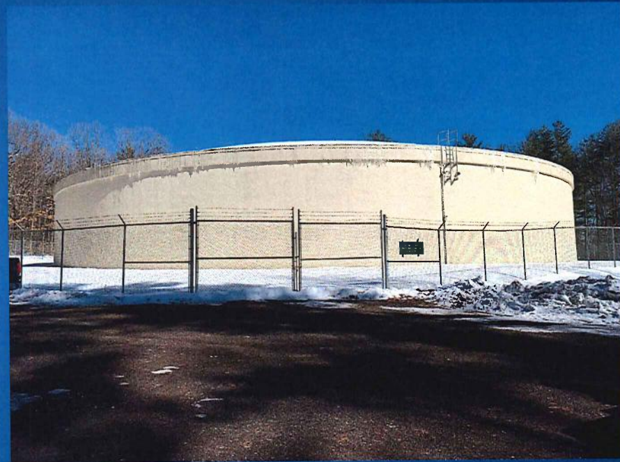
Picture: 4 MG Tsienneto Rd Tank
