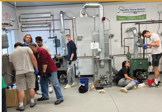
Seacoast area high school students learning the basics of oil heat systems during their last week of class.
