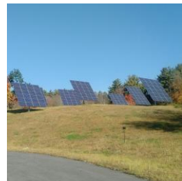
This 86kW solar facility at Derry’s Transfer Station has returned nearly $50,000 in electricity savings since 2018
