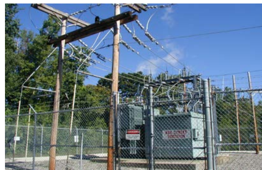
Ash Street Substation
